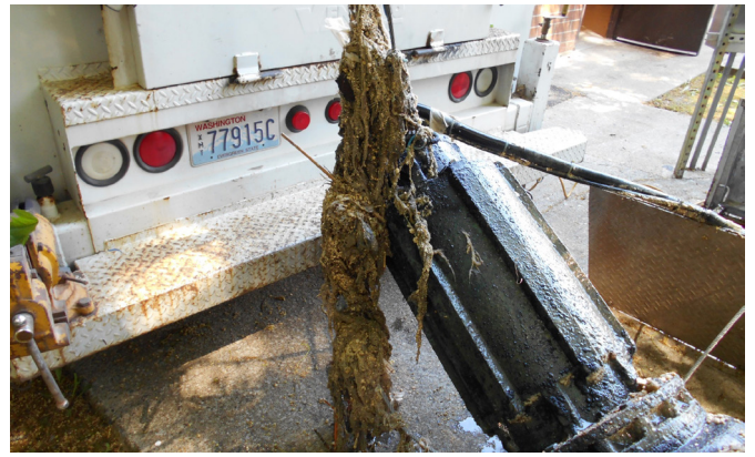
Rags and wipes get caught in the moving components of sewage pumps. They stick together into a single mass, sometimes several feet long.
